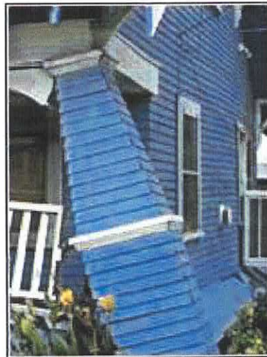
Figure 10 Earthquake Damaged Porch
